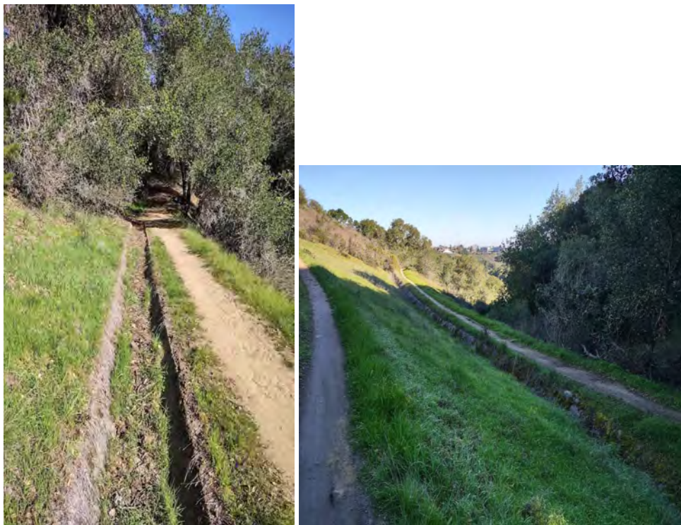
Concrete storm drain culverts along “Flow” trail in need of maintenance.
